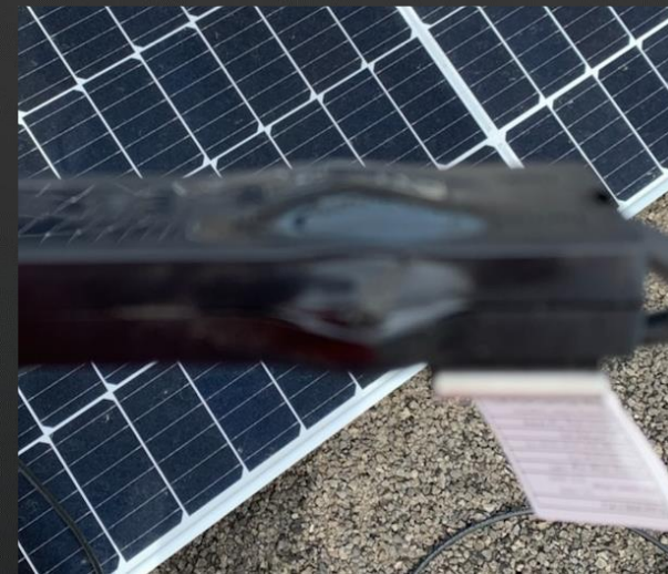
Visual Inspection: Enclosure bubbling
